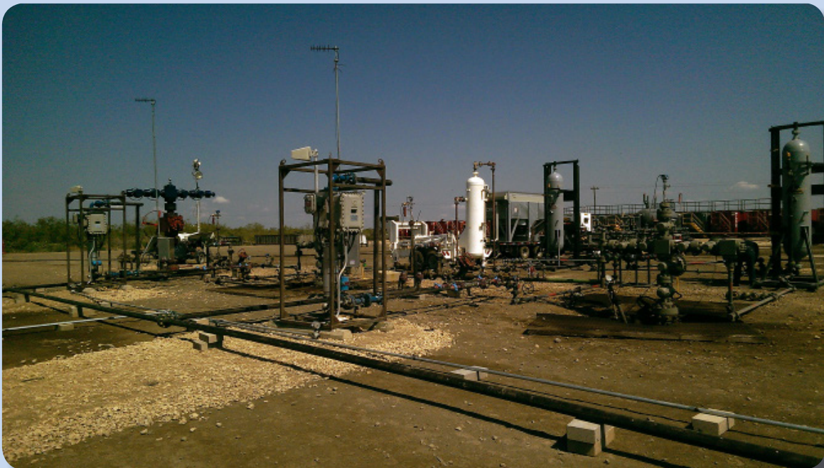
Compact MPFM Installation, South Texas
